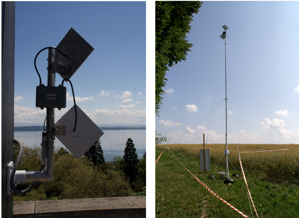
(a) Node01 mounted on the roof top of the University of Neuchâtel.
