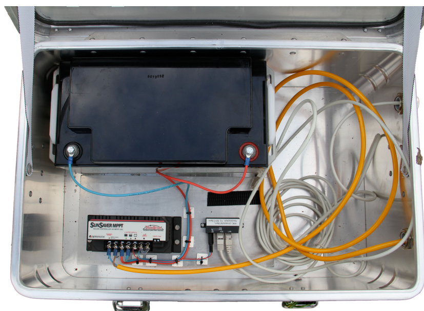
Figure 7: Power supply box with solar charger, acid battery, and passive PoE adapter.
