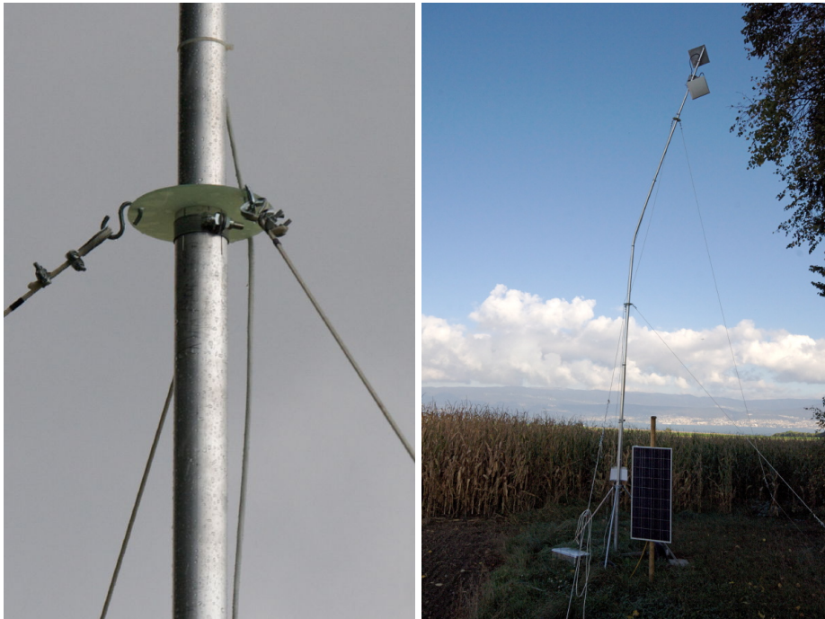
(a) Movable guying clamp to prevent torsion of mast (b) Broken antenna due to strong winds and loose guying (node02)
